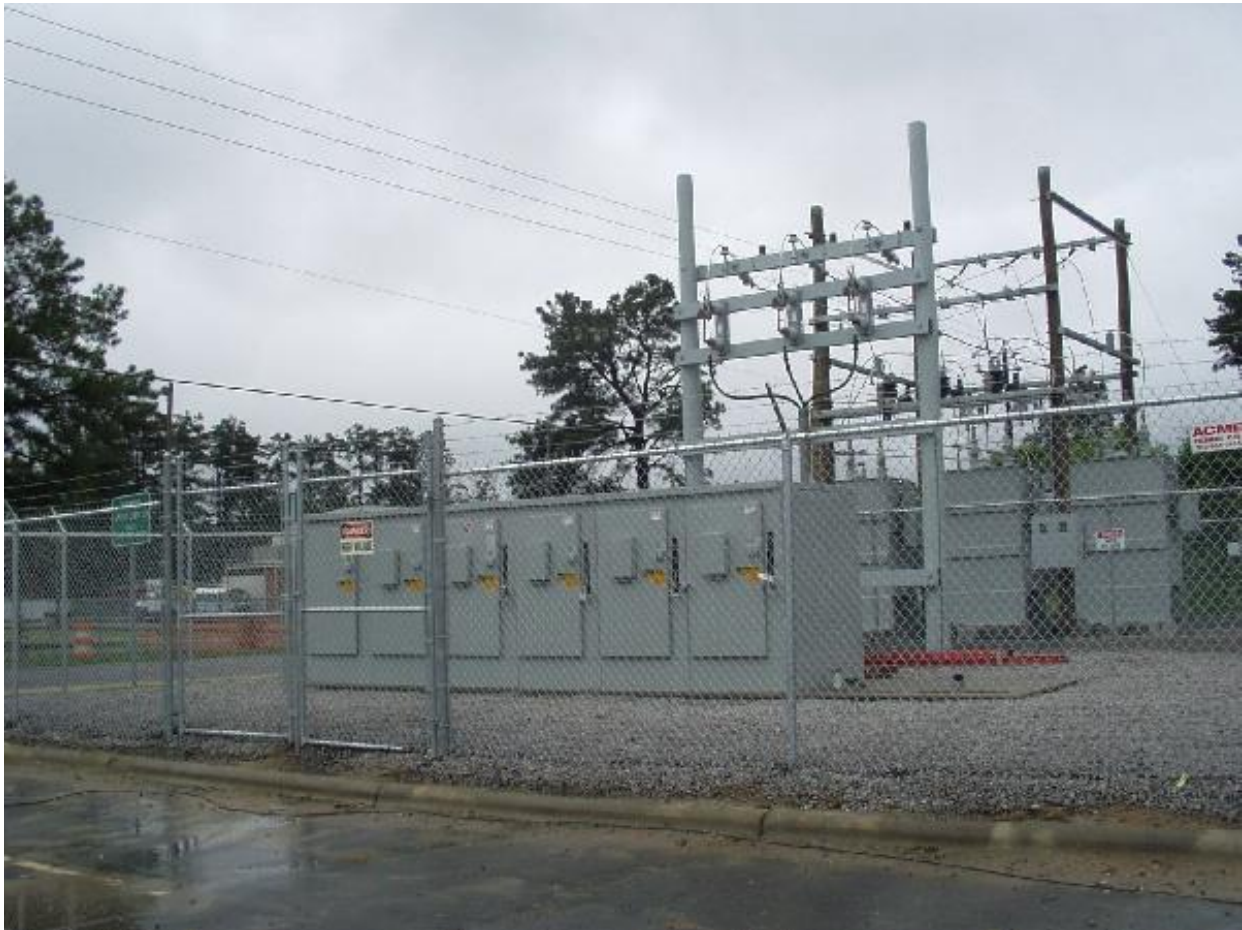
Main UNC Pembroke Substation and Switchgear
